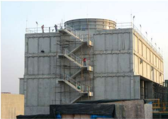
100MW Co-generation Plant Rayong, Thailand
