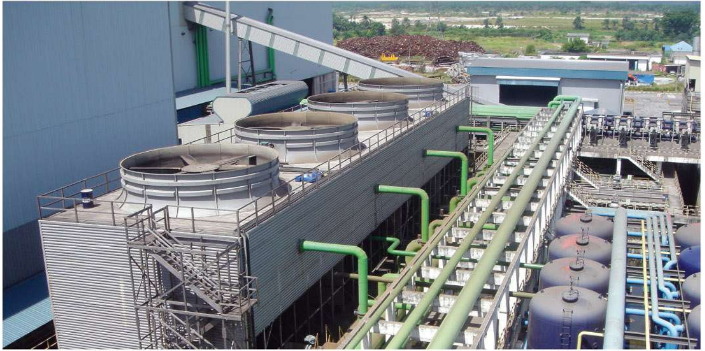
12,000m 3 /hr, Selangor, Malaysia
