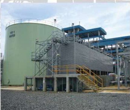
3,000 m 3 /hr, Sandakan Malaysia
