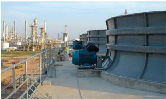
60MW Co-generation Plant Malacca, Malaysia
