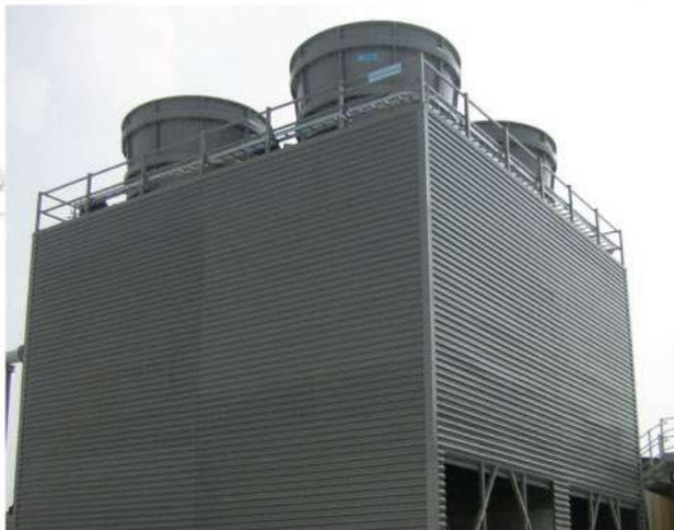
2,000 m 3 /hr, Selangor Malaysia
