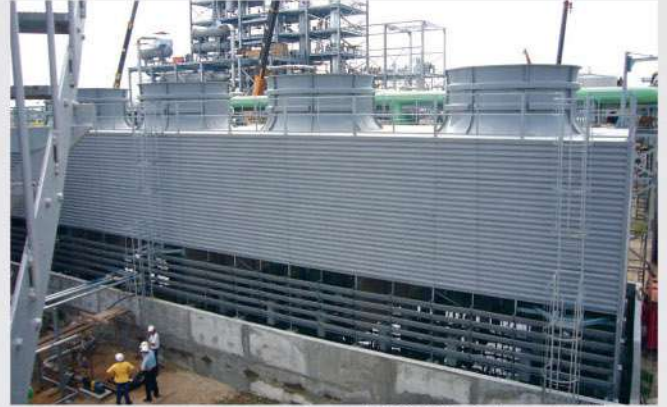
3,000m 3 /hr, Selangor, Malaysia
